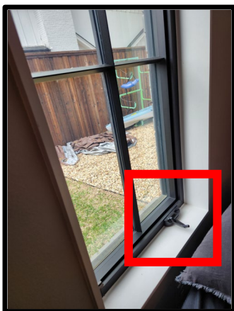
Casement windows with aluminum locking mechanisms.
